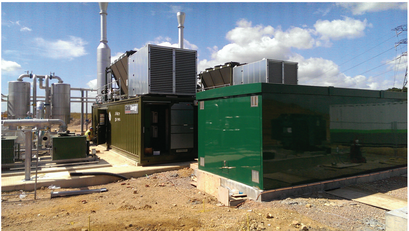
Integral to the new facility will be the engines shown above that convert gas generated by the AD process into electricity for export to the national grid
